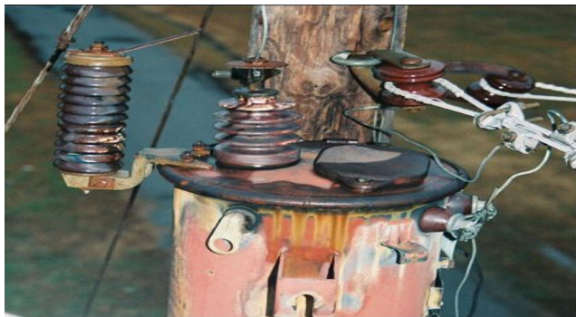
FIGURE 12. Damaged external bushing that caused intermittent faults [3].
