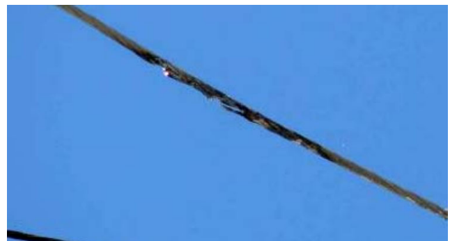
FIGURE 10. Conductor damage from wind-induced conductor slap [3].
