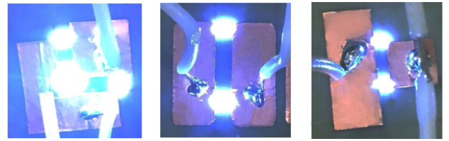
FIGURE 18. Typical location of the observed flashover between the pads for different designs.
