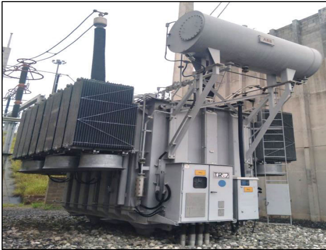
FIGURE 1. Power transformer installed in a substation.
