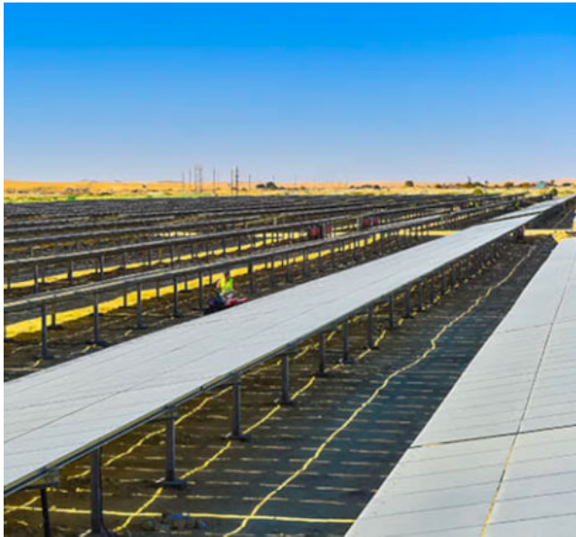
FIGURE 2. Siwa solar station.
