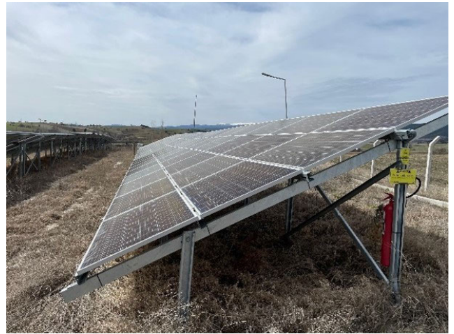
FIGURE 1. Solar power plant image.
