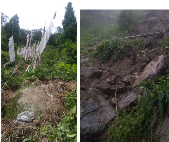
FIGURE 15. Slope instabilities near the site, triggered by rainfall.
