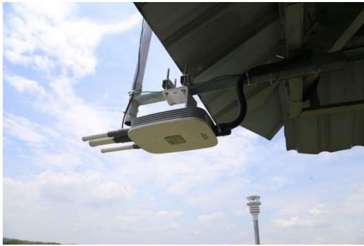
FIGURE 2. LoRa gateway installed on top of the observation tower.
