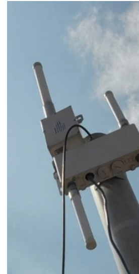
FIGURE 2. LoRa gateway utilized in the setup.
