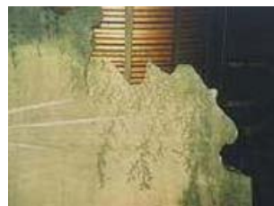
Figure 1. Tree-shaped mark on the pressboard barrier in a scrapped transformer [1].
