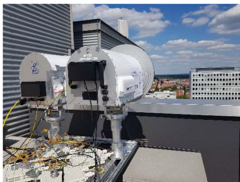
FIGURE 15. 300 GHz ThoR link connecting two buildings at the campus of TU Braunschweig.
