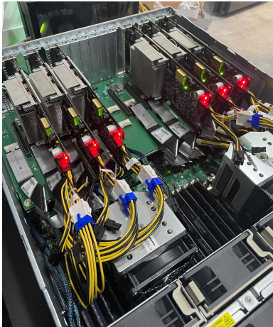
FIGURE 14. Six PCIe cards mounted with the chips and passive heat sinks are plugged into a server.
