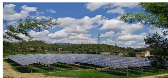
FIGURE 11. Distributed photovoltaic power generation project in Xinlong village, Waxi town, Zijin county.
