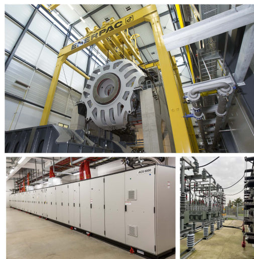
FIGURE 4. Picture of the nacelle test bench hall, converter system, and filter bank at DyNaLab in Bremerhaven.
