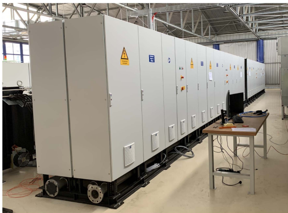
FIGURE 10. Converter cabinets of the PQ4Wind test bench containing a total of 20 MW installed converter power for emulation.
