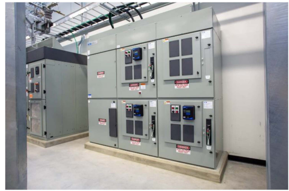
FIGURE 9. 4.16 kV rated eaton ampgard motor control equipment.
