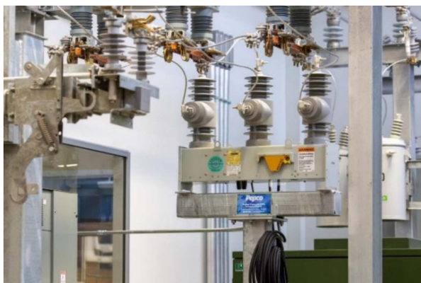
FIGURE 12. Three-phase reclosers and disconnect switches.
