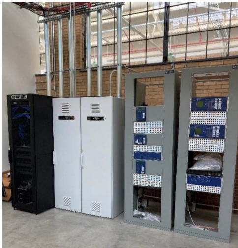
FIGURE 16. Server (left), emerson ovation platform (center), schweitzer relays (right).
