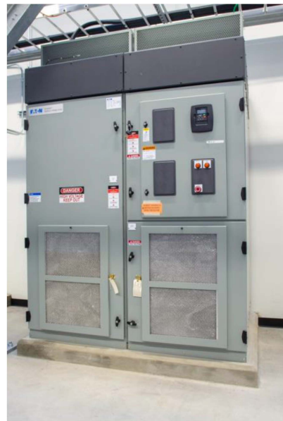
FIGURE 10. 4.16 kV 500 HP MV drive.
