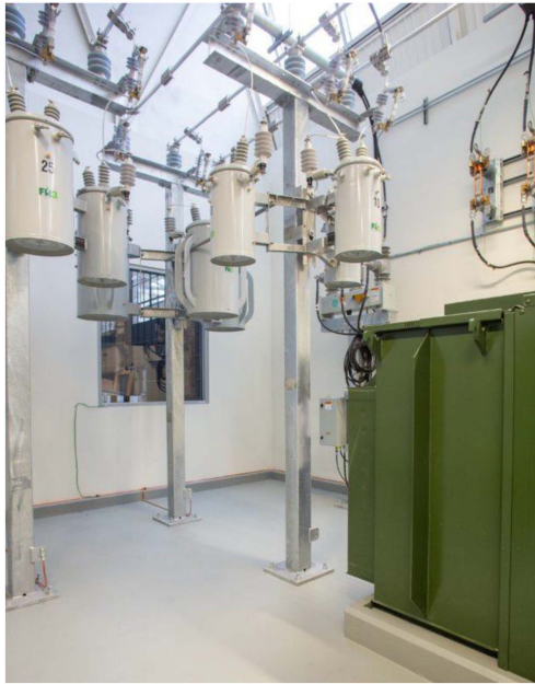
FIGURE 8. Pole-mounted transformers (480 V and 240 V secondary).
