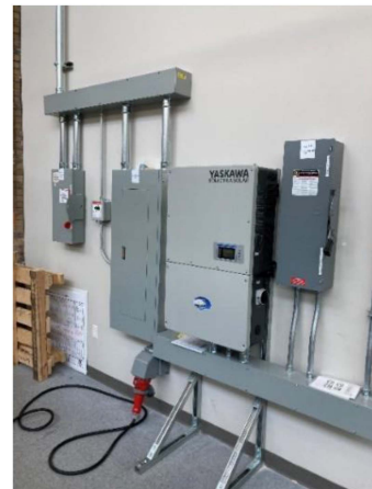
FIGURE 20. AC (far left) and DC (right) transfer switches along with inverter.
