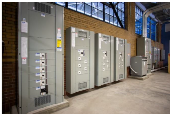
FIGURE 13. 480Vac electrical panels (far right) and DC electrical panels (no electrical feeds entering DC panels currently).
