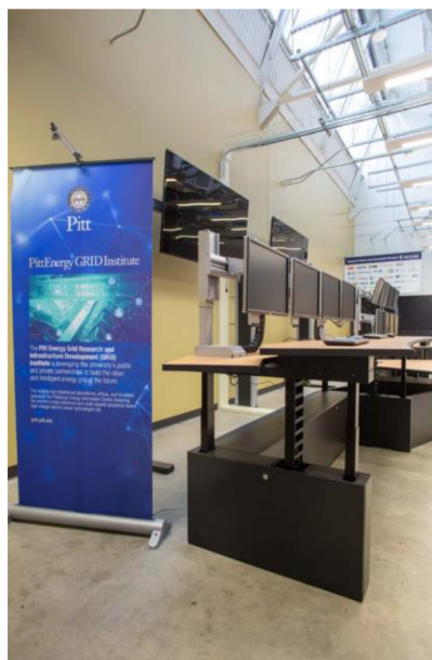
FIGURE 15. Operations center for controlling MV AC equipment.
