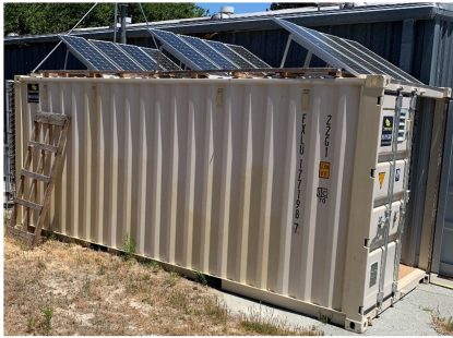
FIGURE 7. Microgrid enclosure and PV arrays.
