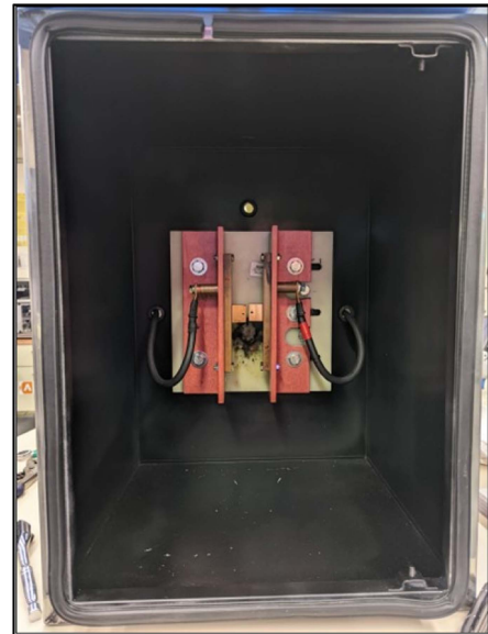
FIGURE 5. UTA enclosure with vertical copper electrodes.
