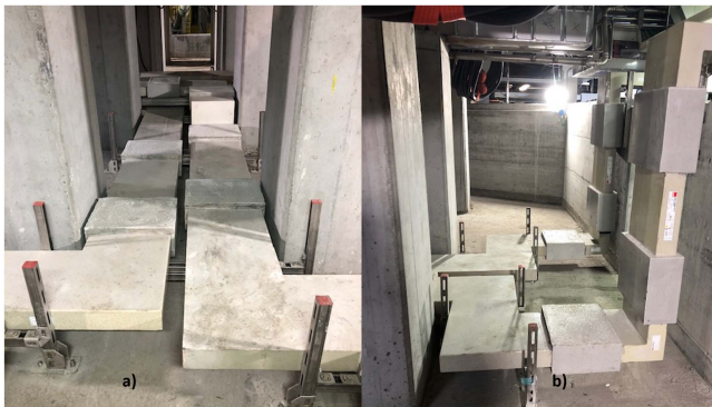
FIGURE 23. Sections of the closure of loops A and C: a) path under the furnace; b) ascent towards the busbar ducts.
