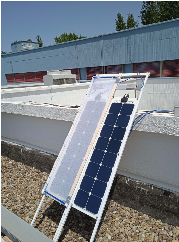
FIGURE 3. PV modules in series using a screen onto one of them to simulate partial shadowing conditions.
