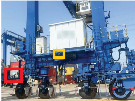
FIGURE 2. RTG platform and camera installation in this study. The red box shows the location where the AXIS P1448-LE or Hanwha XNO-6080R cameras are mounted, with lane lines in both directions. The yellow box shows the Hanwha XNF-8010RVM camera mounting location.
