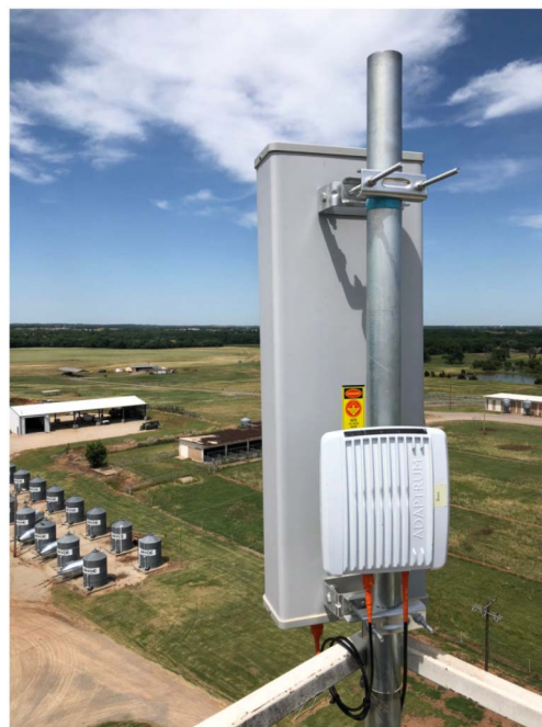
FIGURE 5. Base radio and antenna on OSU feedmill tower.
