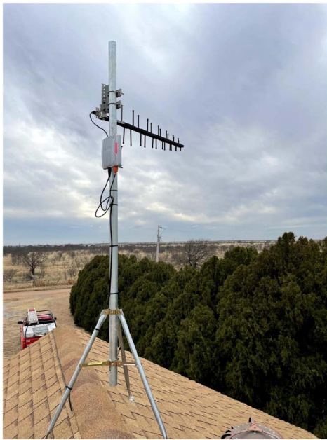
FIGURE 16. Client antenna at rooftop of client premises at Tillman County.
