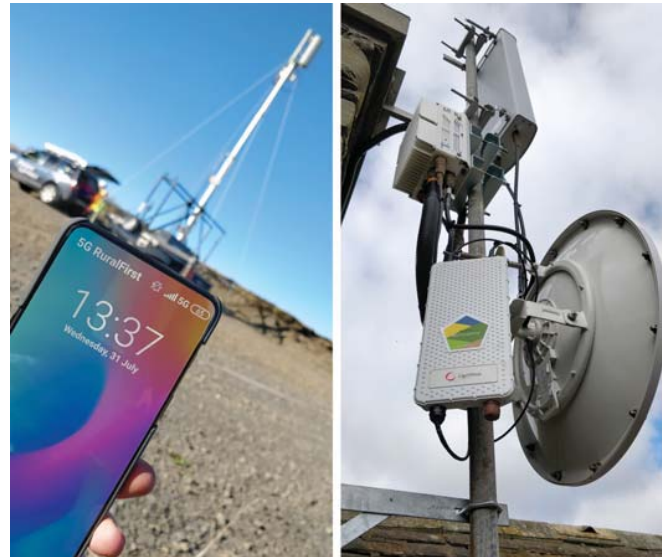
FIGURE 1. Photographs of shared spectrum mobile basestations from the 5G RuralFirst project. (Left) a trailer mounted generator-powered pneumatic mast system with 5G cell and on-board core network, and (right) close-up of a 700 MHz radio head and 5 GHz microwave backhaul at a remote rural site.
