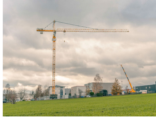
Fig. 1. Experimental tower crane Liebherr 154 EC-H Litronic 6, which is utilized on common construction sites. ©IntCDC, University of Stuttgart.
