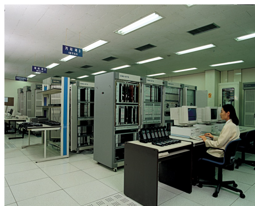
Fig. 3. CMS prototype installed in ETRI
