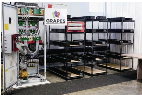
Fig. 19 CHB cabinet-level implementation
