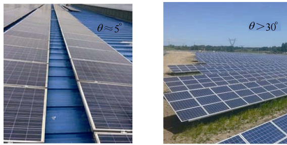
(a) PV panel on the roof (b) PV panel on the ground Fig.17 PV panels in two typical applications
