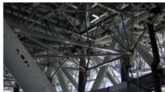
Figure 22b. A rear view of a panel unit installed in the backup structure of the LMT. The segments of about 5 m size are supported at their corners on the backup structure by motorized adjusters.
