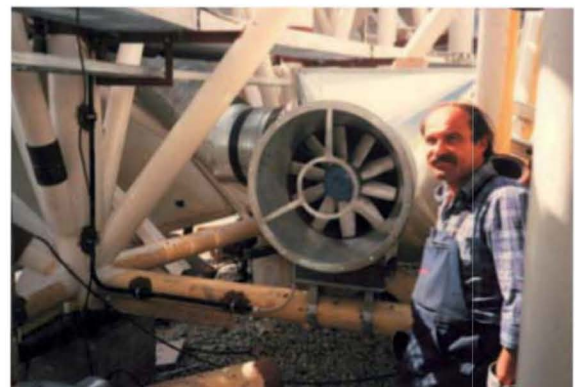
Figure 15b. One of the five ventilators that cause a circulating air movement with controlled temperature through the backup structure. This structure is covered on the outside by a cladding of thermal insulation panels, visible in the upper picture.
