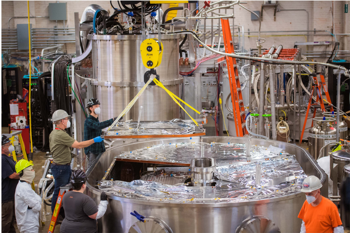
Fig. 7. Installation of the final panel of the main cryostat radiation shield prior to the 20-T campaign. The TFMC is visible underneath. MLI blankets cover the exterior surface of the radiation shield, including ports.
