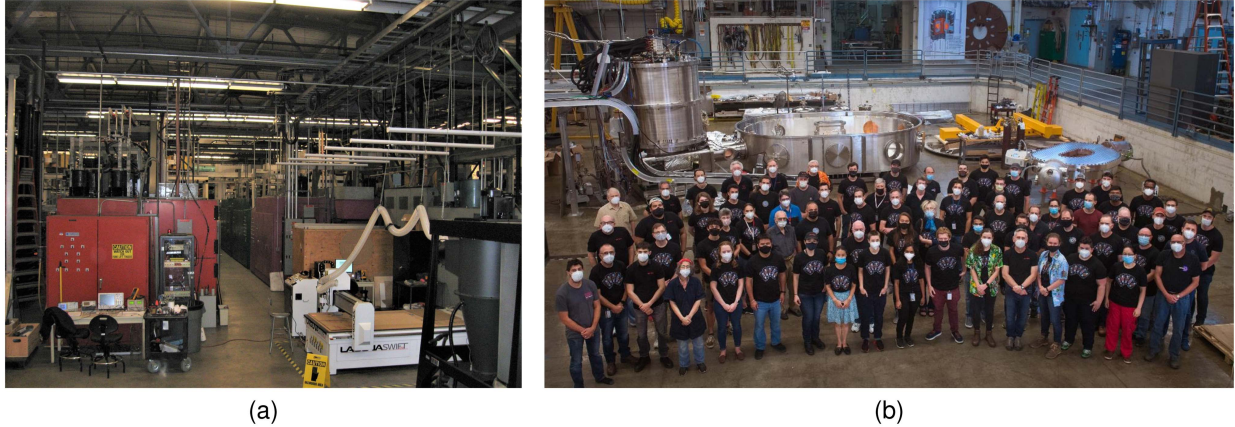
Fig. 1. (a) C-Mod “Power Room” in late 2019 prior to its transformation into the magnet test facility and (b) the same space in July 2021, just prior to the installation of the TFMC into the main cryostat, shown with the majority of the PSFC and CFS personnel involved in the PSFC project.
