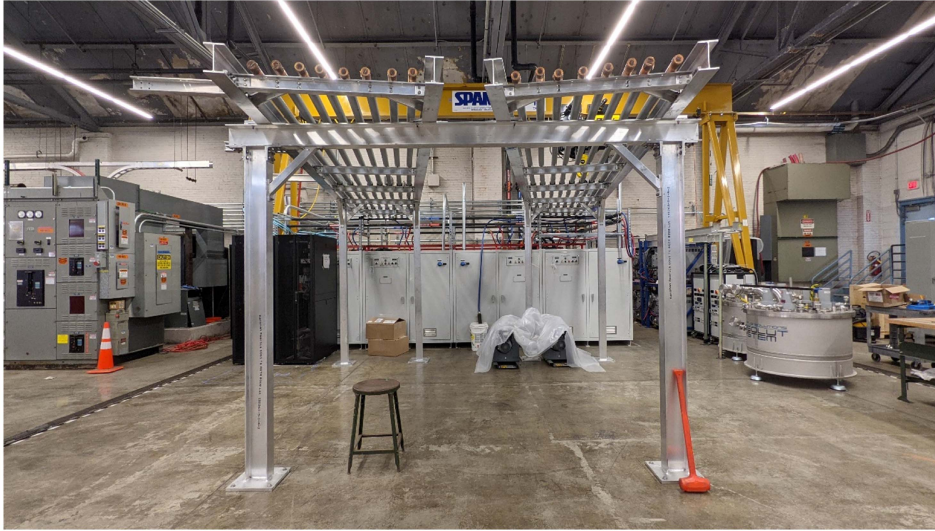
Fig. 14. Photograph of 16 water-cooled bus lines newly arranged on stand, prior to installation of plumbing; supply and return for each cabinet are adjacent.
