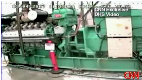
FIGURE 2. Screen capture showing generator used in the Aurora test.
