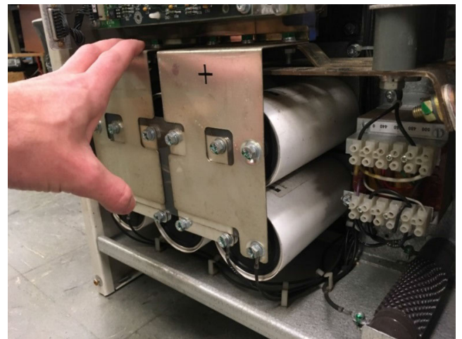
FIGURE 15. DC link capacitors on 100 hp inverter.
