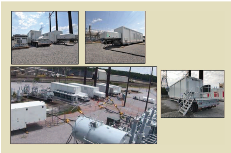
FIG 4 Four photographs showing FACTS equipment, including a cooler bank, converters, and reactor trailer. The photographs are related to the presentation by David Roop of Dominion Energy titled “FACTS: Flexibly Solutions for a Changing Grid.” (Photos courtesy of Dominion Energy.)
