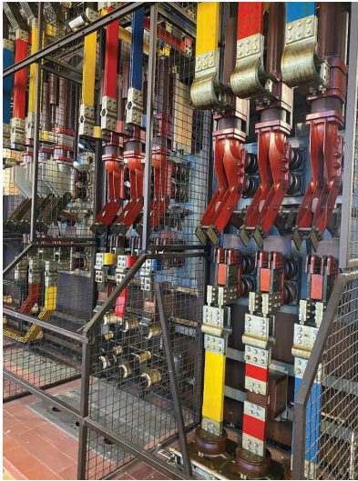
Figure 7. Details of switchgear cabinets at the C Mine industrial museum, Genk.
