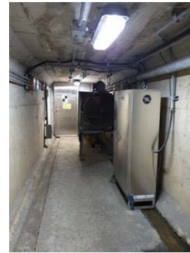
FIGURE 12. Control box installation status near exhaust fan no. 6 that affects the exhaust flow.
