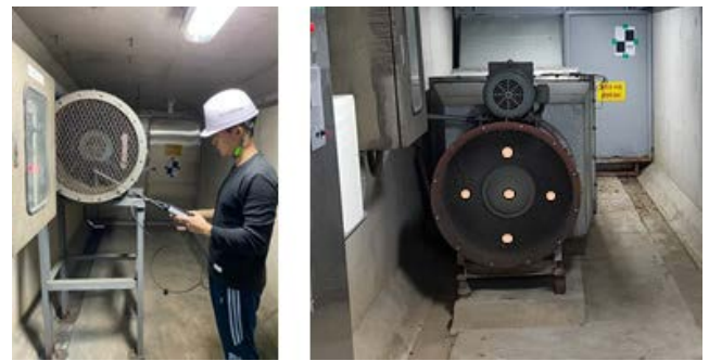
FIGURE 4. Flow velocity measurement experiment at the inlet of exhaust fan (○: measurement point).
