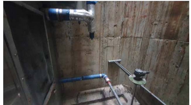
FIGURE 3. Insufficient space in the external part of the inlet vertical duct for fan capacity measurement.
