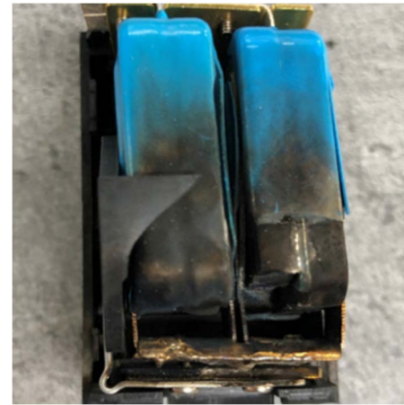
FIGURE 2. SPD damaged by thermal runaway.
