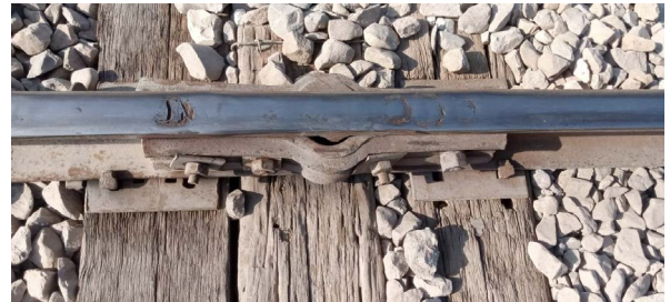
FIGURE 10. Wheel Burn on railway track.
