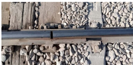
FIGURE 14. Low joint fault.
