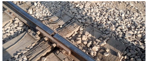
FIGURE 11. Creep fault on railway track.
