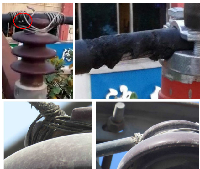
FIGURE 2. Partial discharge problem and burned insulation on covered conductor in Inland areas.
