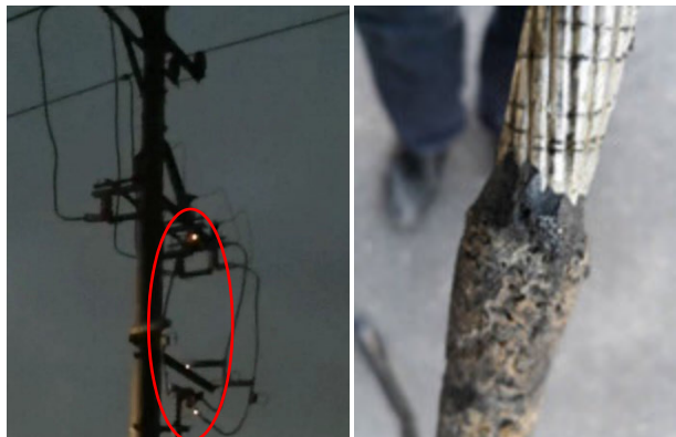
FIGURE 1. Partial discharge problem and burned insulation on covered conductor in Coastal areas.
