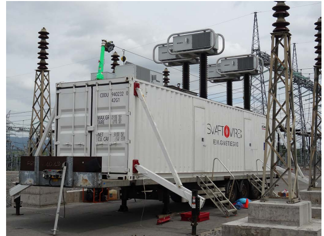
FIGURE 7. MPFC parked inside the substation and four MPFC modules fully elevated to their installation position.
