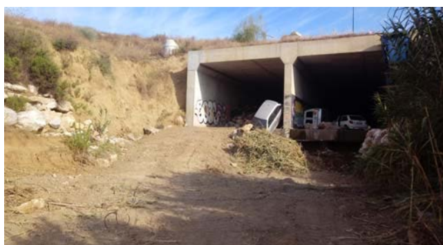
FIGURE 8. Tunnel entrance with wrecked vehicles.
