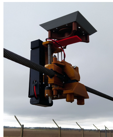
FIGURE 29. The recharging station installed on the power line at the airport on the real power line setup.
