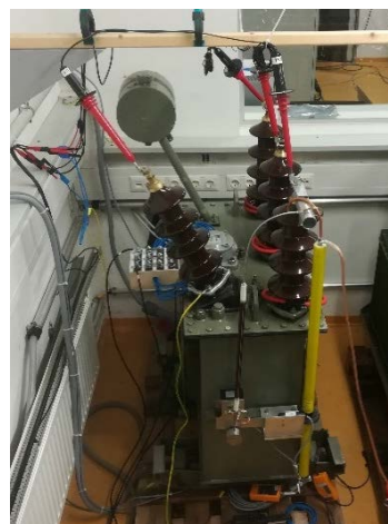
FIGURE 2. Transformer under test.
