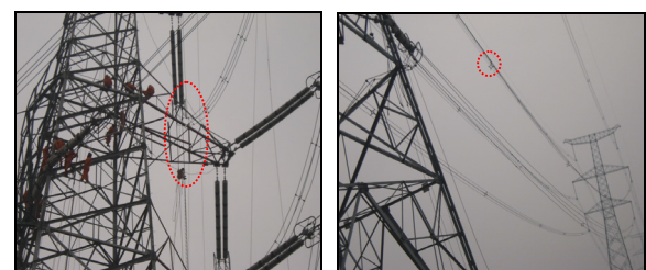
(a) Damage of the tower arm; (b) Damage of the spacer
