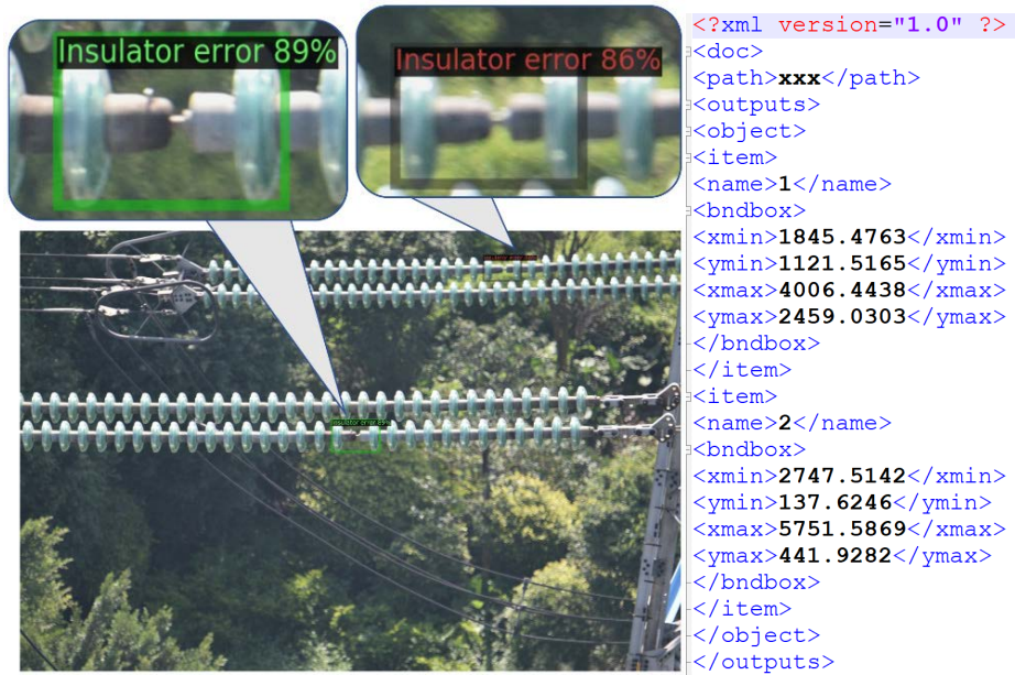
FIGURE 9. Identification and location of insulator defects.
