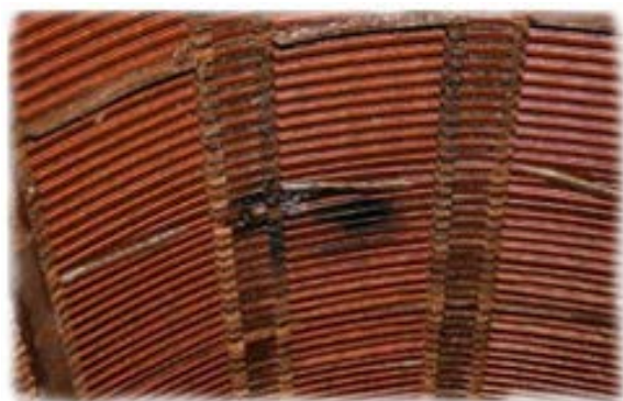
FIGURE 1. Transformer winding breakdown caused by overheating.
