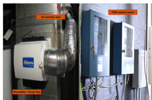
FIGURE 9. Humidification plant (a) supply air (SA) fan (b) return air (RA) fan (c) the VFD installed.
