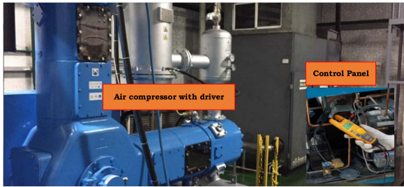
FIGURE 6. Condition monitoring of compressor units-measurement of energy consumed using Fluke power analyzer.
