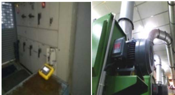
FIGURE 8. Testing of existing electric motors through motor control centre panel and installing new IE 3 motors.
