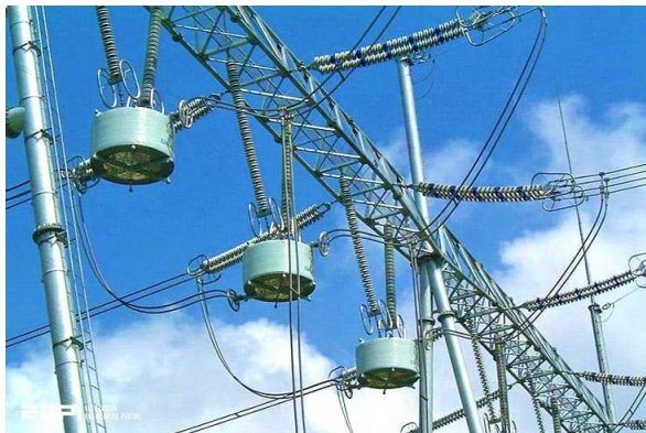
FIGURE 6. An example of powerline communication (PLC) systems in power transmission and distribution [68].
