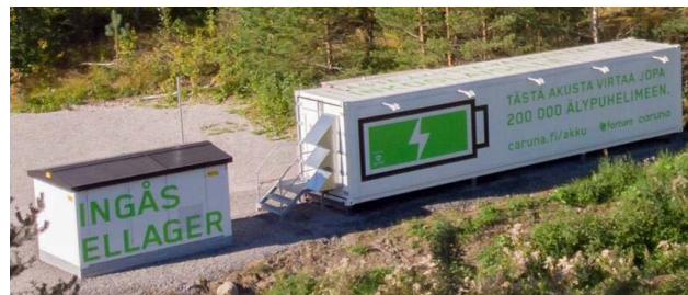
FIGURE 9. 1 MVA Battery energy storage system installed in Ingå, Finland.
