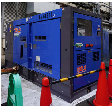
FIGURE 5. 125-kVA diesel synchronous generator.
