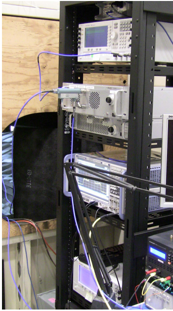
FIGURE 9. Waveform generator and transmitter connected to a high-power amplifier with cables leading to the antenna located in the adjacent anechoic chamber.
