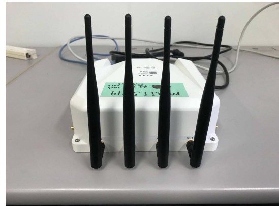
FIGURE 4. Example of WLAN access point.
