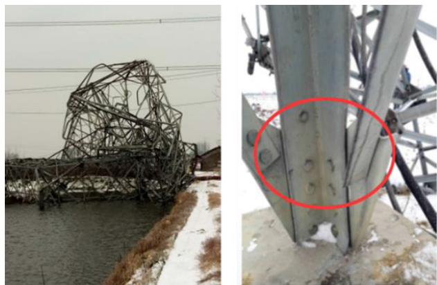
FIGURE 3. 141# iron tower inverted tower.
