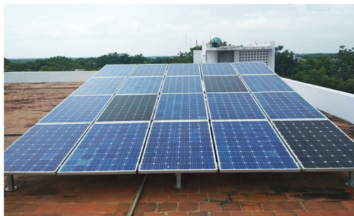
FIGURE 5. 5kWp PV system for the experimental verification.
