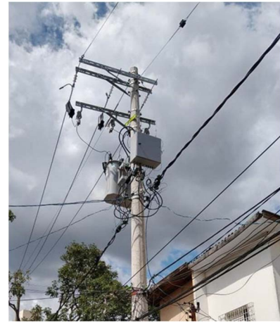
FIGURE 16. LVC field installed.
