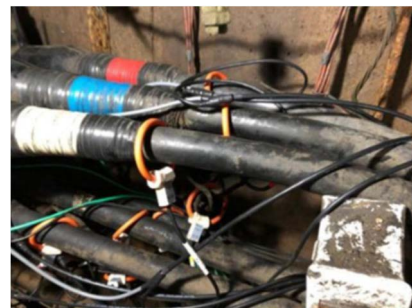
FIGURE 23. Current sensors in underground distribution grid, Underground Fault Tracking.
